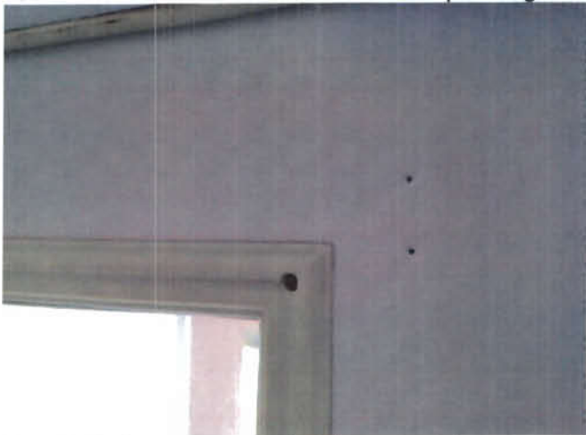
Certain holes were not filled / repaired before painting.
