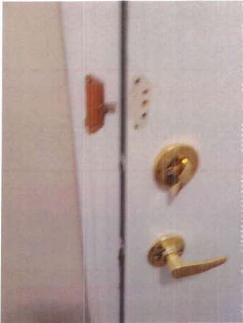
Qaiser removed some hardware after painting and failed to re-attach it.
