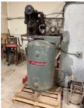
Industrial 5HP Compressor
