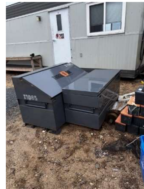
G-03 Generator Skid 8kw Diesel
