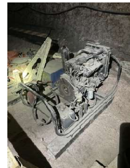
G-03 Generator Skid 8kw Diesel
