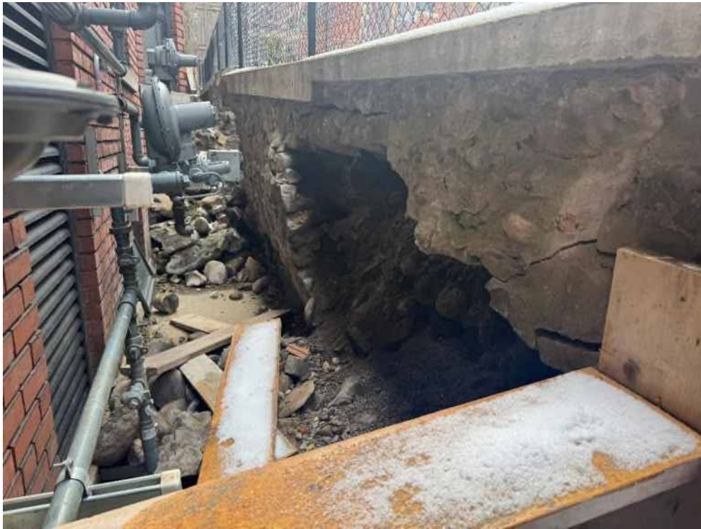
Retaining Wall Failure
